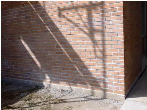
23, 24. Poor tuck pointing
