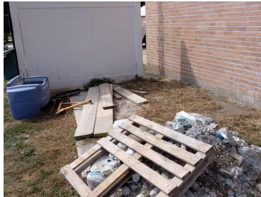
14. Debris left on site
