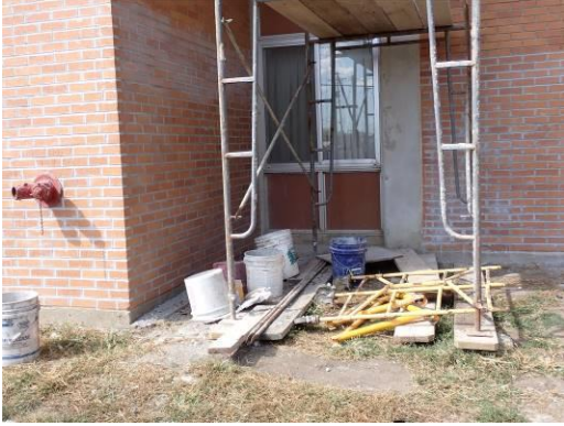
15, 16. Scaffold left on site
